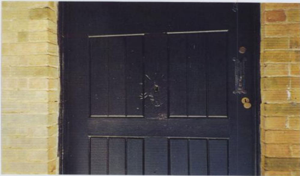
VANDALISM TO GATE HOUSE
